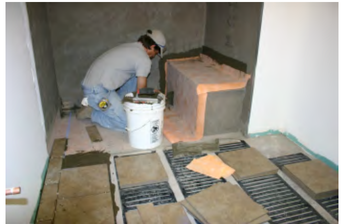
Heating on the floor and the bench
