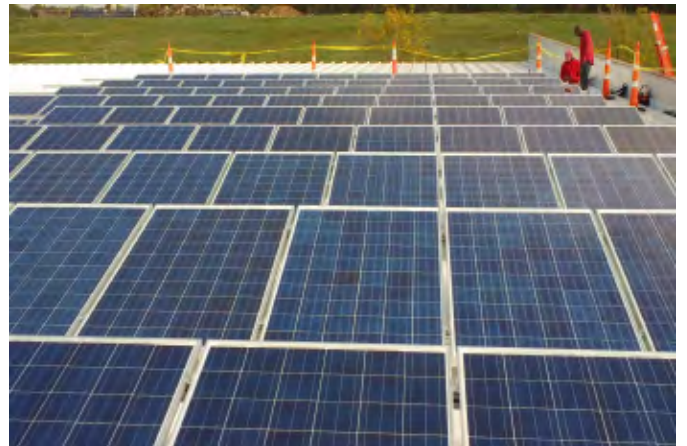
Solar Panles on Roof
