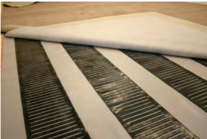
Elements on insulated concrete between two layers of carpet cushion and under carpet
