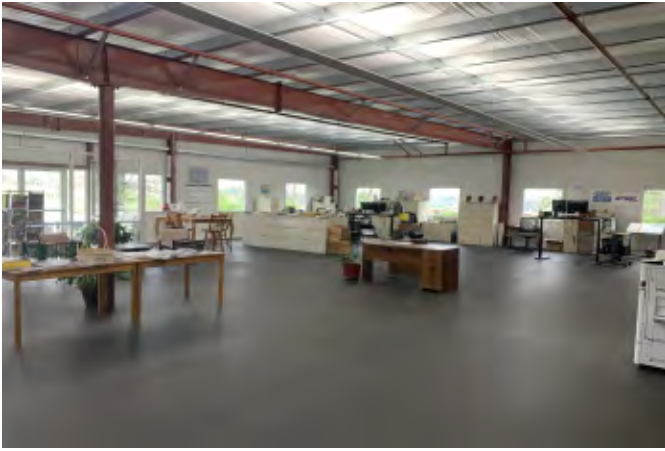
Open Office - Elements in Concrete and Under Rubber Mats
